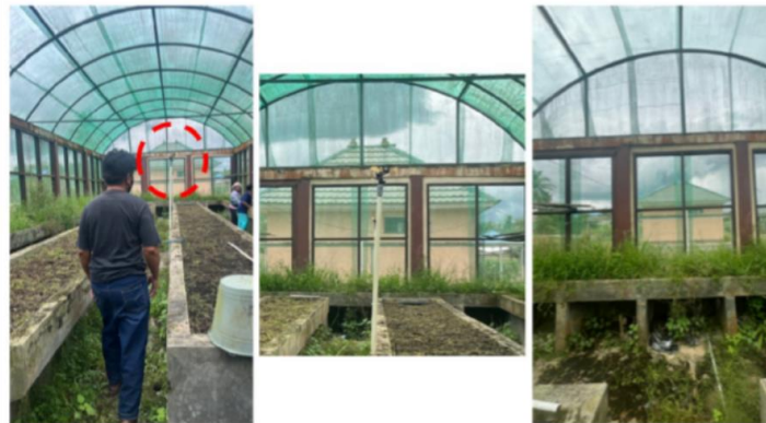
Figure 2. Initial condition of the TTP greenhouse showing the sprinkler system causing uneven water distribution and inefficient irrigation.
